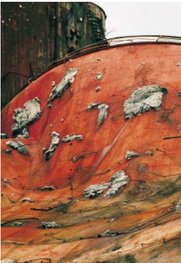
Destroyed oil tank at Novi Sad
